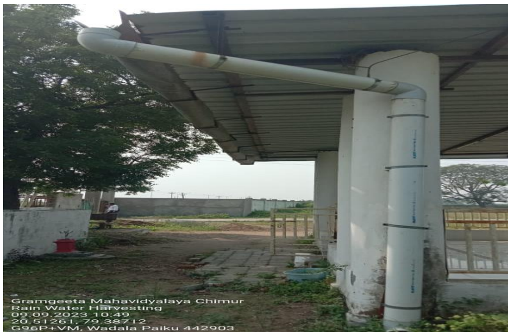
GEOTAGE PHOTO: RAIN WATER HARVESTING UNIT
